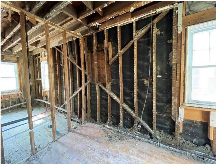
Photo 01: View of the existing exterior wall framing at the north side of the building. Note discontinuous wall studs and lack of base plates at interior wall framing.
