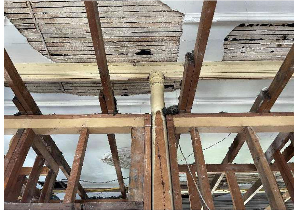
Photo 06: View of a structural wood column that supports the roof framing. Note that column is compromised.
